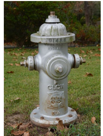
A fire hydrant.
