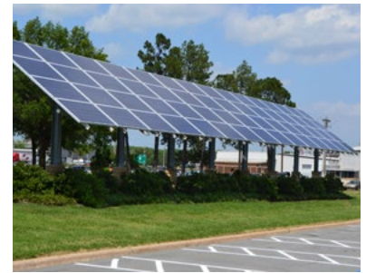
Ground-mounted solar panels.
