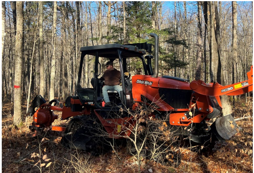
Trenching an oak wilt pocket in Pigeon River Country with a vibratory plow.
