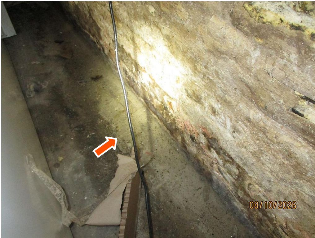
Photo 13: Masonry sediment on floor adjacent to foundation wall
