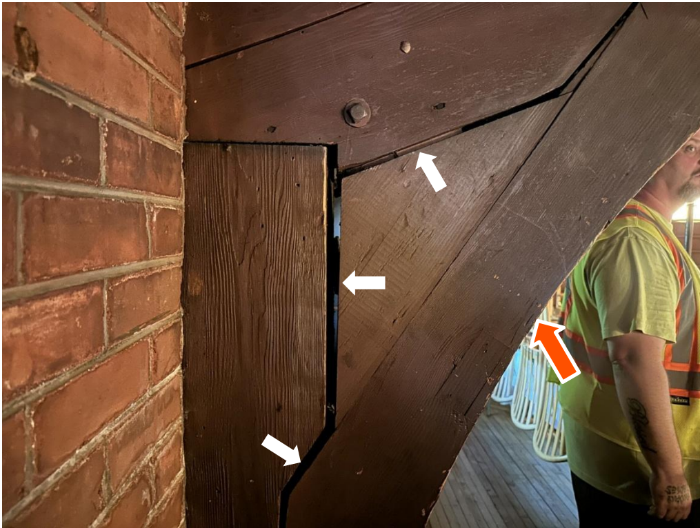
Photo 7: Gap between knee brace (indicated with orange arrow) and column and roof girder
