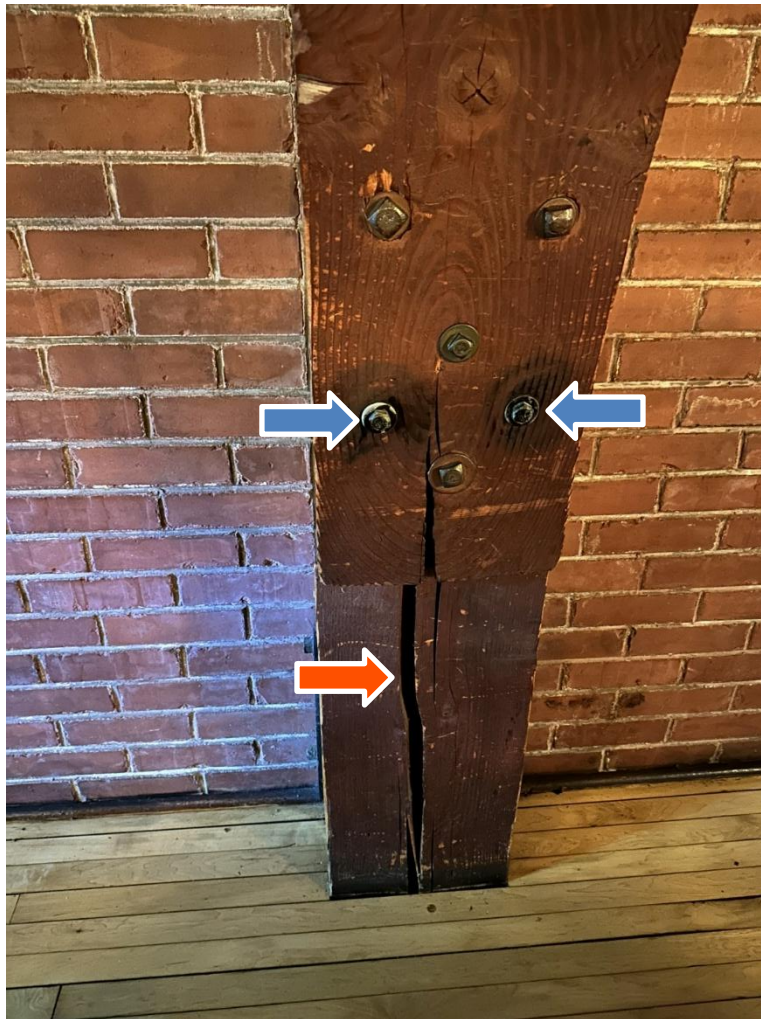
Photo 8: Orange arrow indicates checks in wood column. Blue arrow indicates two newer bolts. The older bolts have square heads.
