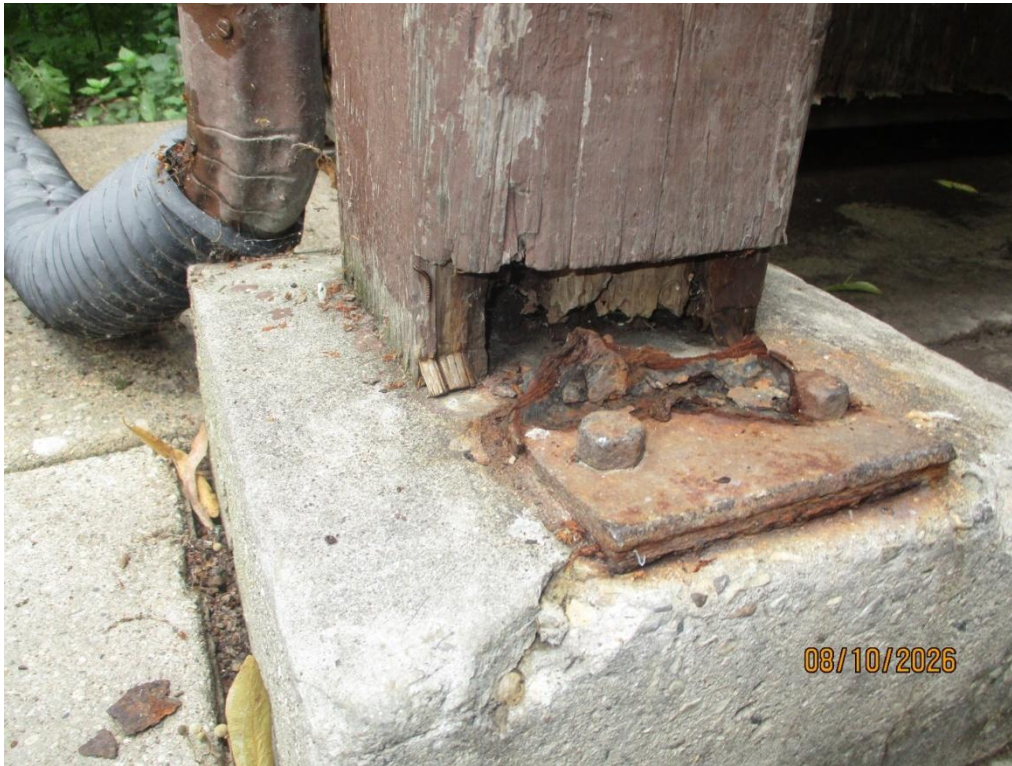
Photo 5: Corroded steel angle
