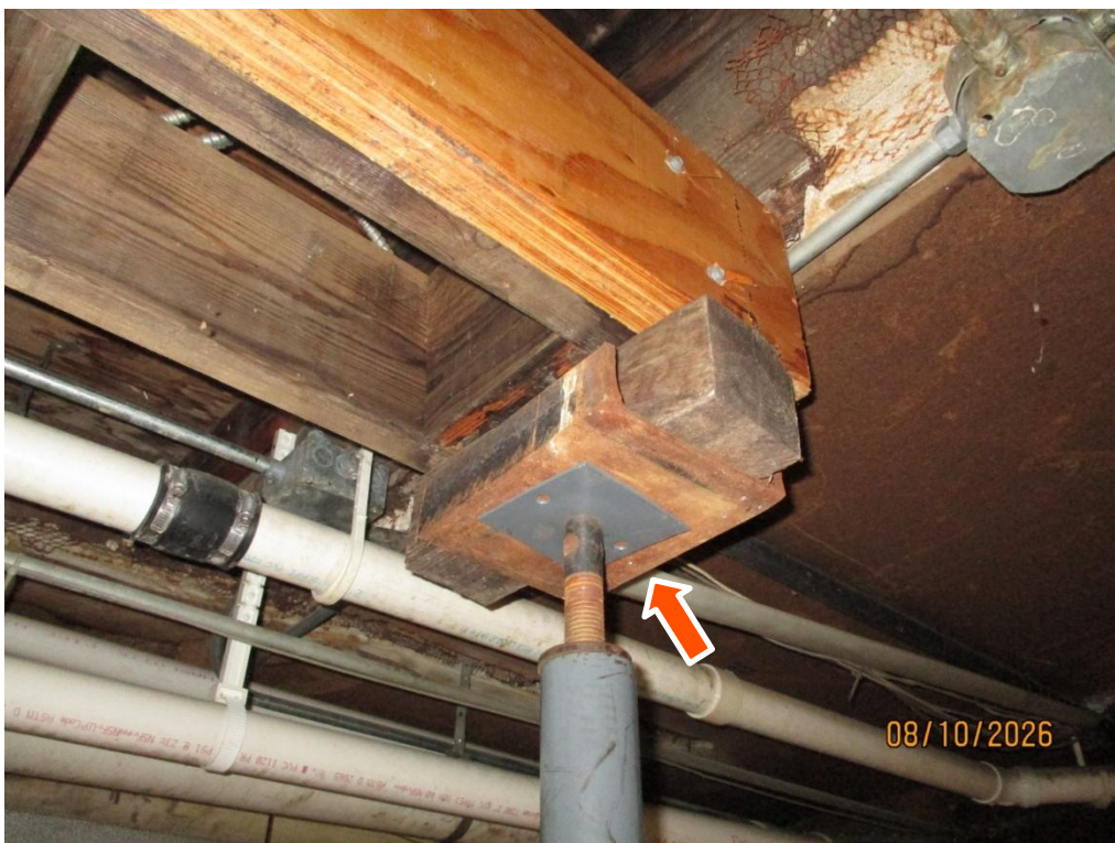
Photo 10: The top of the shoring is not mechanically attached to the supported framing
