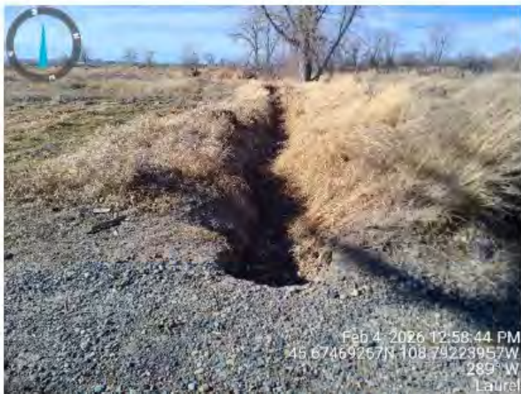
BED-AND-BANK-2, REPRESENTATIVE PHOTO
